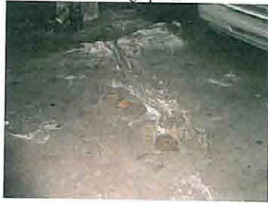
Basement Floor Drain 4630 Broadway, New York, NY
